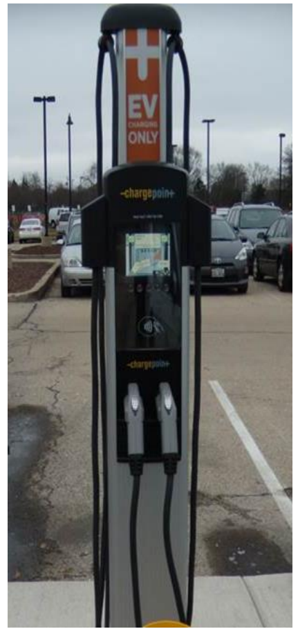
EV CHARGING STATION
